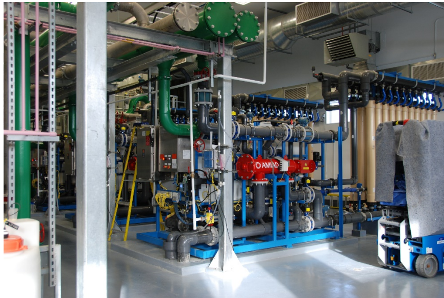
Nano Filtration Membrane System
