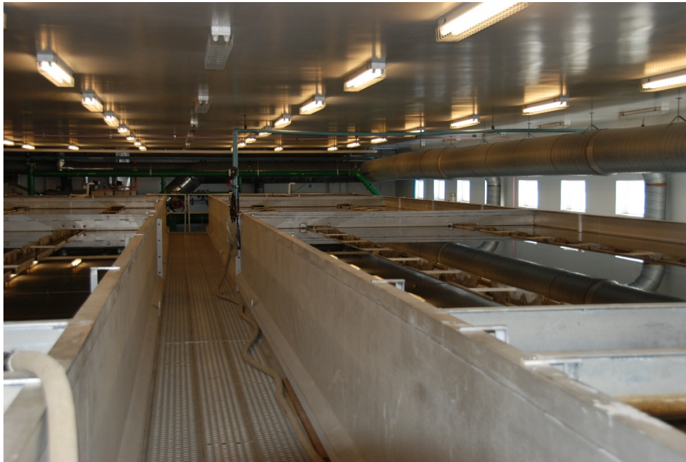
Pre Treatment Trains
